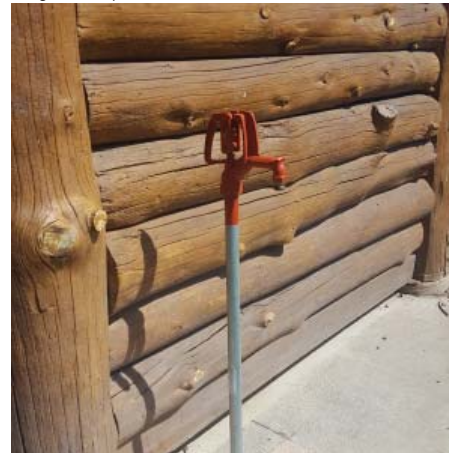
Image 68: Potable water hydrant at Eagle Park
