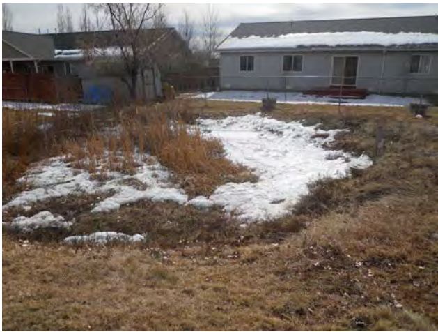
Photo 28 – Pond 28 - Heavily Silted w/Vegetative Growth
