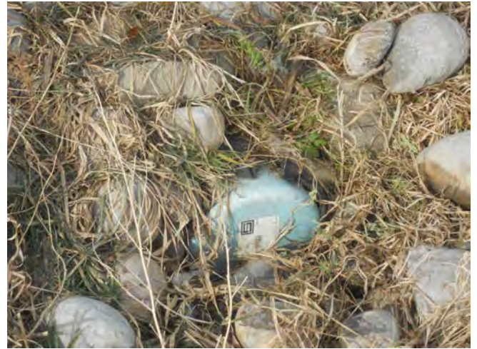
Photo 12 – Pond 6 – Outlet Pipe Obstructed
