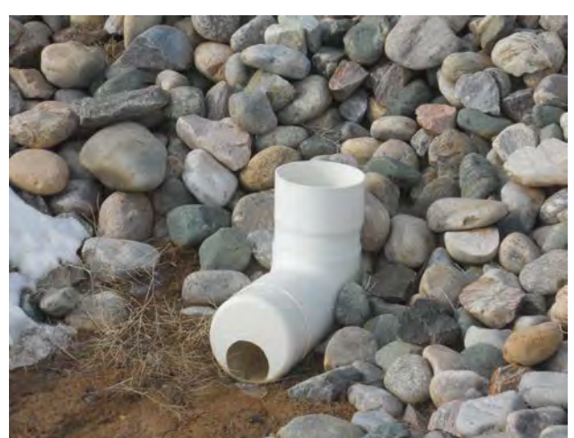
Photo 14 – Pond 8 – Outlet Pipe/Weir
