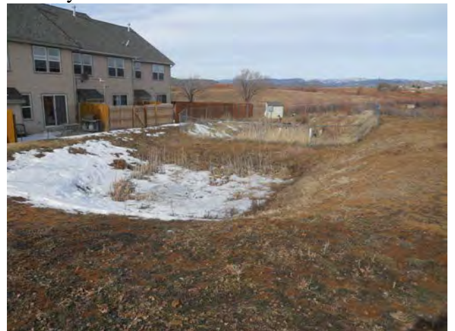
Photo 20 – Pond 21 – Pond is Heavily Silted, Outlet pipe Not Visible, Significant Vegetative Growth
