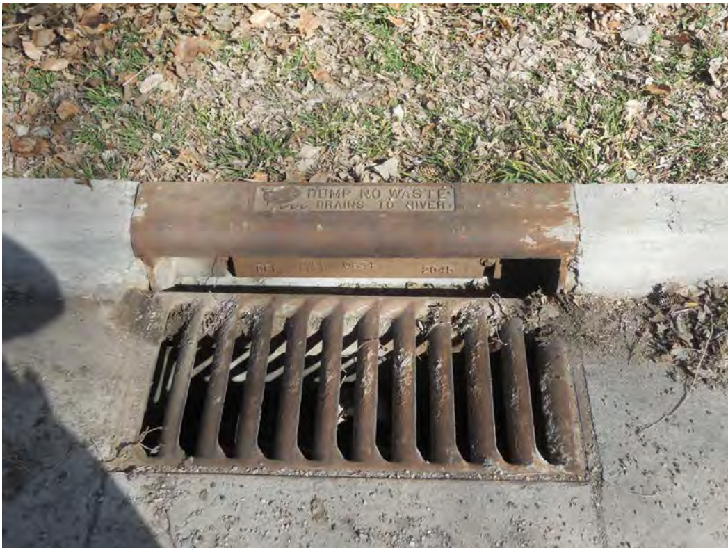
Photo 4 – Inlet – Single, 3-Ft Standard Cast Iron, (CI) w/Capture Vanes
