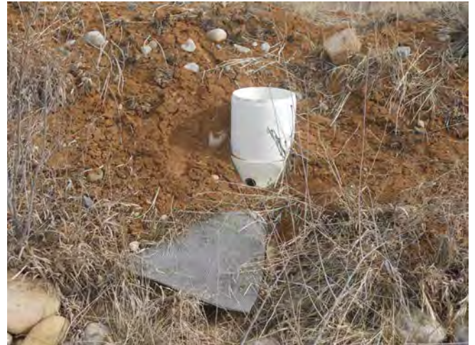
Photo 30 – Pond 41 – Outlet Pipe
