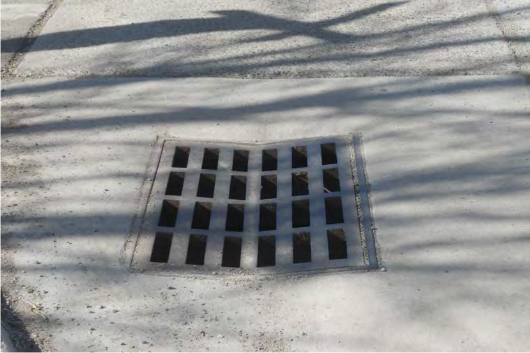
Photo 5 – Inlet – Single, 2-Ft X 3-Ft, Parallel Vane in a Sump Configuration
