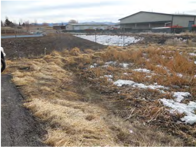
Photo 15 – Pond 9 –Heavily Silted with Significant Vegetation Growth, Outlet Pipe Located Approximately Near Center of Pond, Overgrown
