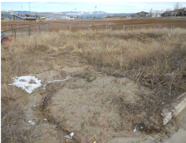
Photo 16 – Pond 10 - Heavily Silted with Significant Vegetation Growth, Outlet Pipe Silted Over/Not Visible
