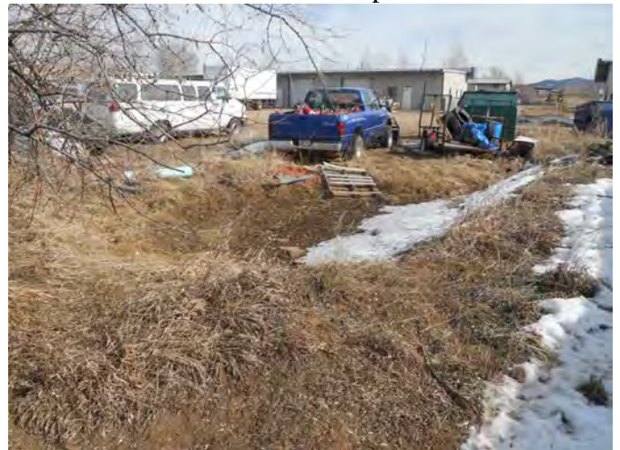
Photo 26 – Pond 26 – Heavily Silted, Debris and Vegetation in Pond
