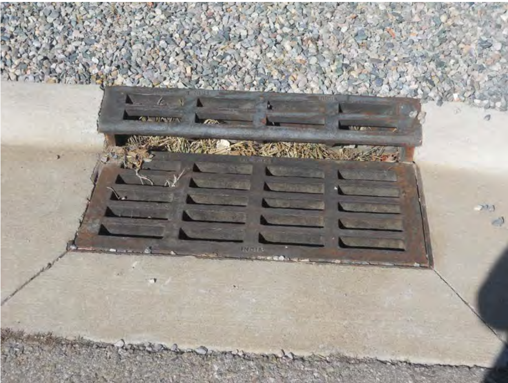
Photo 6 – Inlet – Single, 3-Ft Standard Cast Iron (CI), w/Parallel Vanes
