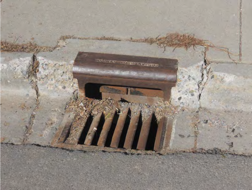
Photo 1 – Inlet – Single, 18-inch, w/Capture Vane
