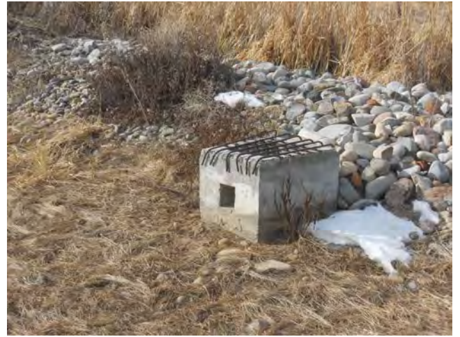
Photo 18 – Pond 11 – Outlet Structure, Containment Berm is at Approximately Same Elevation as Top of Outlet Structure
