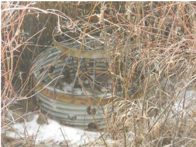
Photo 10 – Pond 2 – Outlet Structure, Vegetation Obstructing Flow to Structure
