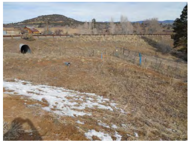
Photo 19 – Pond 18 – Outlet Pipe Near Top of Containment Berm and Appears to be Heavily Silted
