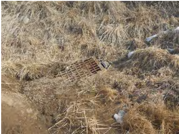
Photo 23 – Pond 25 – Inlet Pipe Obstructed
