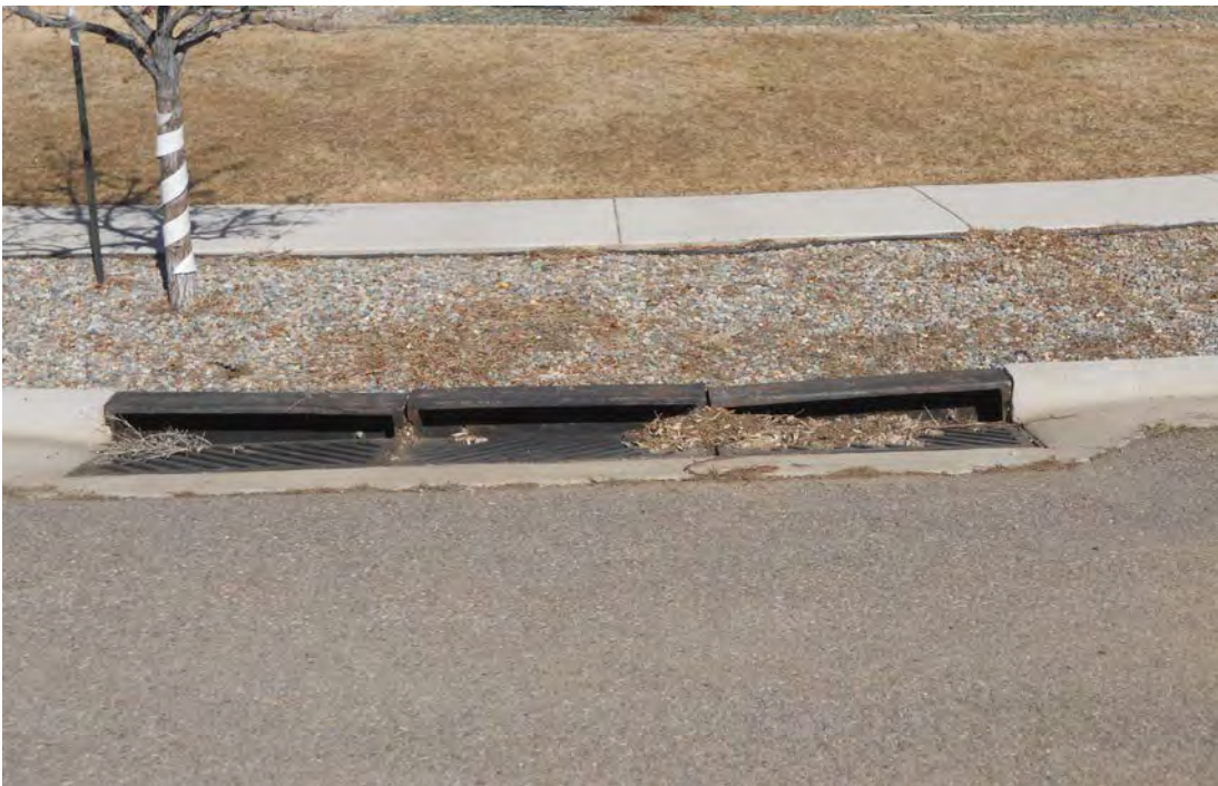
Photo 8 – Inlet – Triple, 3-Ft Standard Cast Iron (CI), w/Slanted/Angled Vanes
