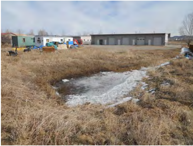
Photo 27 – Pond 27 – Heavily Silted w/Vegetative Growth
