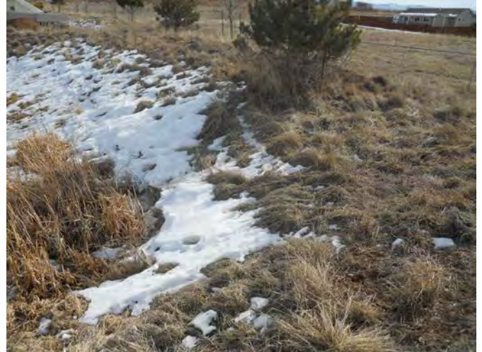
Photo 25 – Pond 25 – Outlet Pipe
