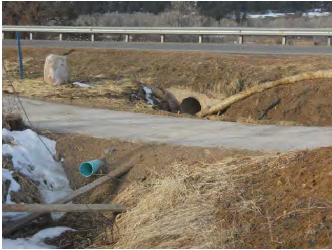
Photo 9 – Pond 1 – Outlet Pipe Near Top of Pond Rim – Debris in Front of Outlet Pipe
