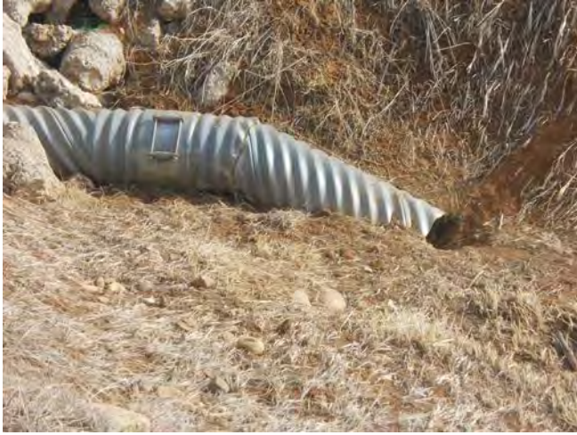
Photo 21 – Pond 23 – Outlet Pipe
