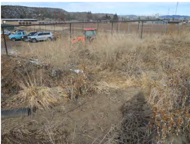
Photo 17 – Pond 10 - Heavily Silted with Significant Vegetation Growth, Outlet Pipe Silted Over/Not Visible, Pond Spills Over Into Adjacent Property
