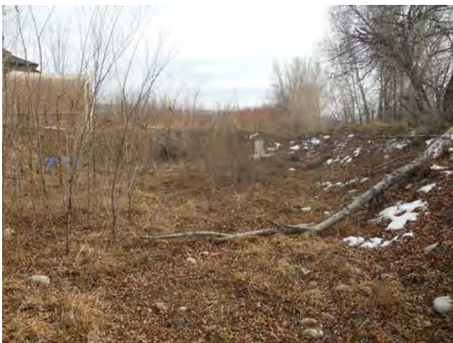
Photo 29 – Pond 34 – Vegetative Growth, Including trees and Debris
