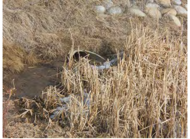
Photo 24 – Pond 25 – Pond Outlet Pipe Silted, Pond is Silted w/Heavy Vegetative Growth
